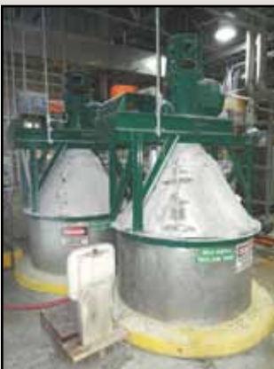
COATING KITCHEN – PARTIAL VIEW
