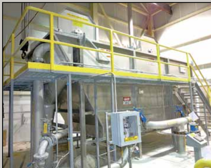
POSEIDON DAF CLARIFIER
