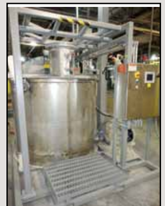
COATING STARCH MAKEDOWN UNIT
